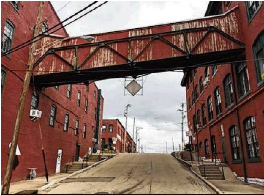
A connecting structure is found between two of the buildings in the Front Street complex, above East Second Street.
